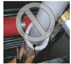
Insulation that does not fit—too loose
